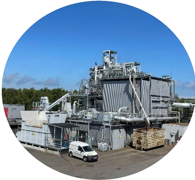
The WoodRoll® plant in Höganäs
