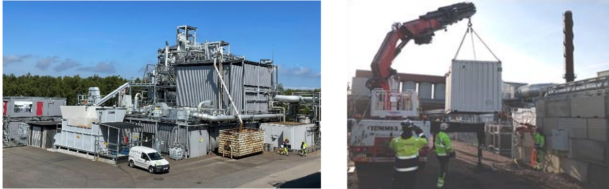
Figure 4. Left: The WoodRoll® gasification plant. Source: Courtesy of Cortus. Right: The biological methanation plant is lifted in place. Photo: Jörgen Held
