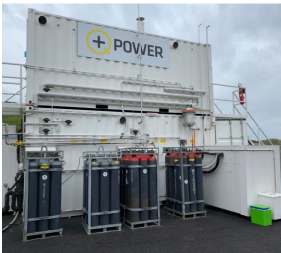
Figure 2. Q Power Oy's mobile biological methanation pilot plant.
