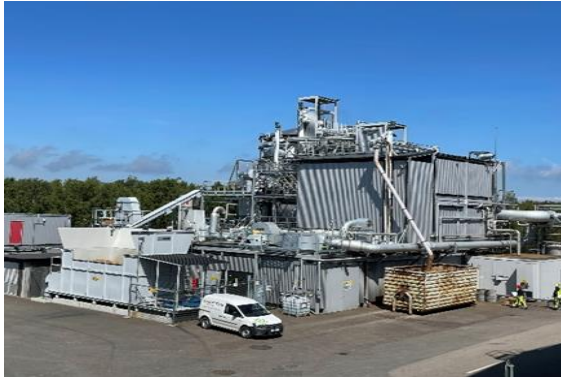
Figure 1. The 6 MW syngas WoodRoll® installation in Höganäs.
